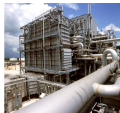
Air Products亚瑟港德克萨斯制氢厂。图片来源：Air Products and Chemicals, Inc.
